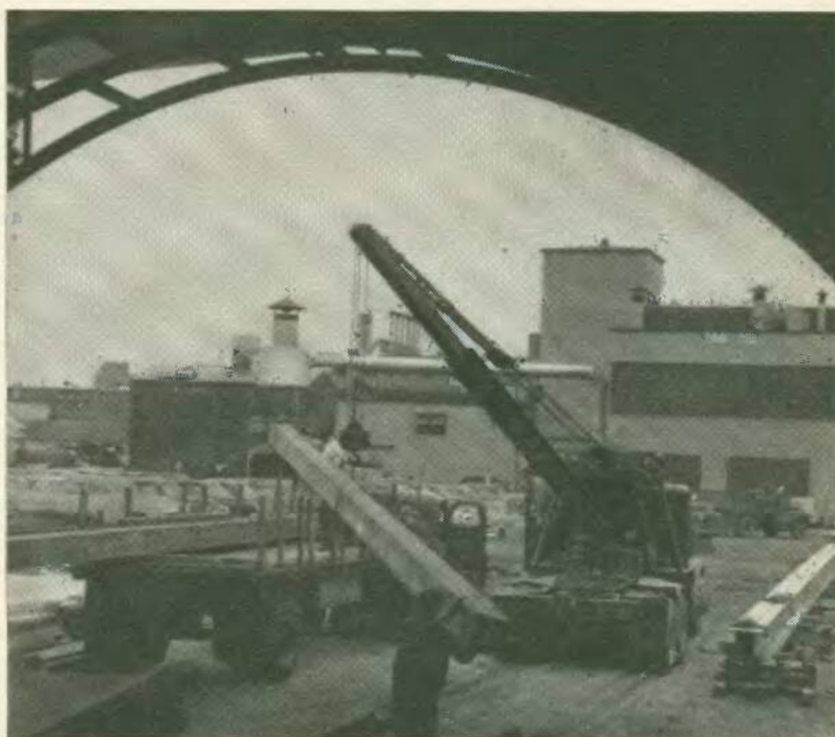
KEEP YOUR EYE ON THE FORWARD LOOK! Multi-million dollar construction begins the greatest Engineering and Design facilities expansion in the company's history. Purpose: to keep bringing you cars demonstrably better than any others.
